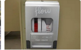
New Period Product Dispensers Installed In All Girl Bathrooms
