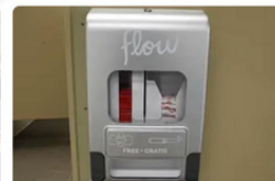
New Period Product Dispensers Installed In All Girl Bathrooms
